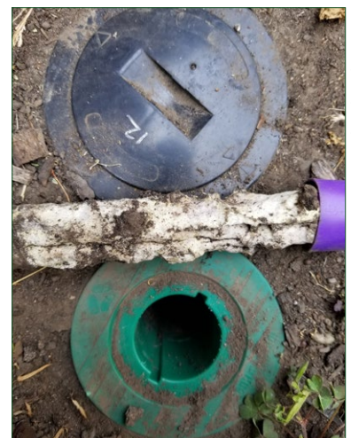
Figure 2. Sentricon Always Active bait tube damaged by termites (with adjacent black monitoring station) approximately 6 months after installation at a single-family home research site in Berkeley.
