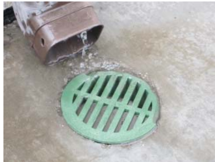
Figure 1. Patio landscape drain located at the base of a roof downspout.
