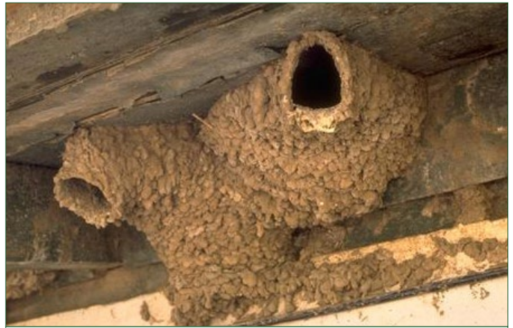
Figure 2. Two mud cliff swallow nests under the eaves of a building.
